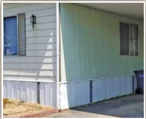
This type of panel skirting around a mobile home unit can become compromised. Fix/patch using methods described in this pamphlet anytime there is damage.
