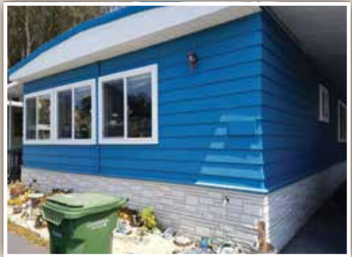
These types of sidings are less conducive to rodent problems, but all vents should still be checked and maintained to prevent rodent entry.
